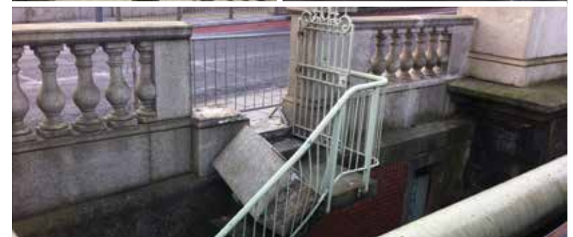
(top): The Old Bridge undergoing reconstruction in 1914; (middle left): one of the ornamental lanterns due for renovation in 2014; (middle right): inspection of the Old Bridge; (above): damage to the Old Bridge in November 2012.
